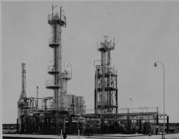
Lube oil and wax hydrofinishing units
