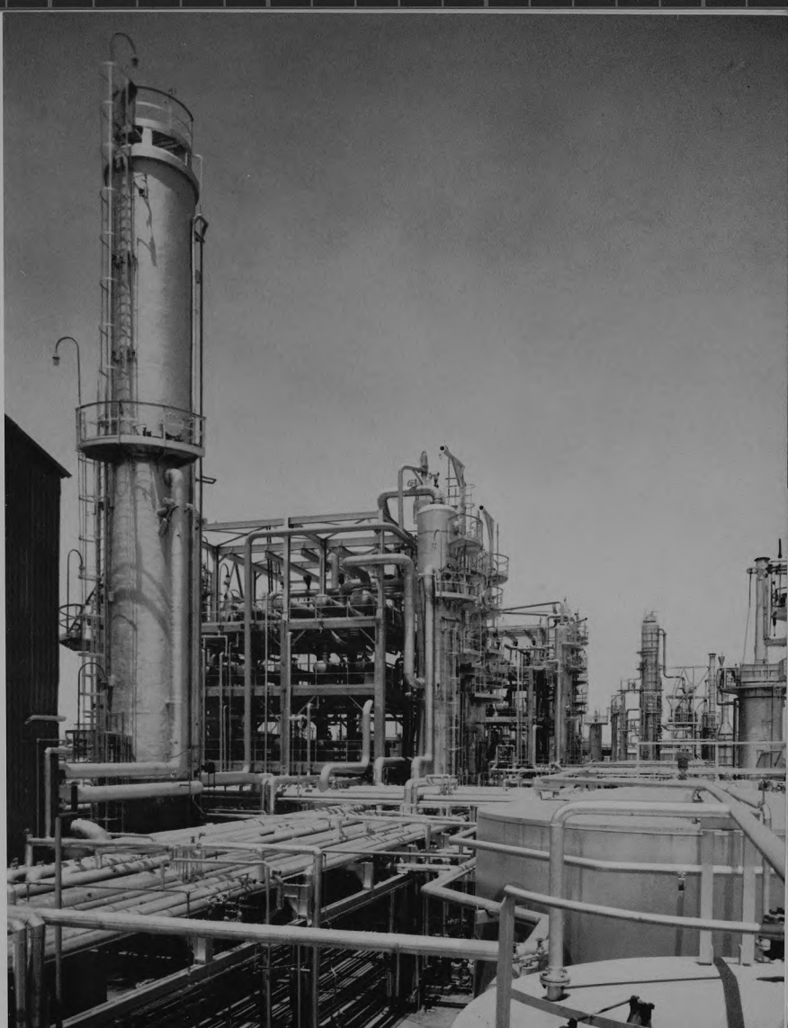
MEK dewaxing and deoiling unit - partial view
