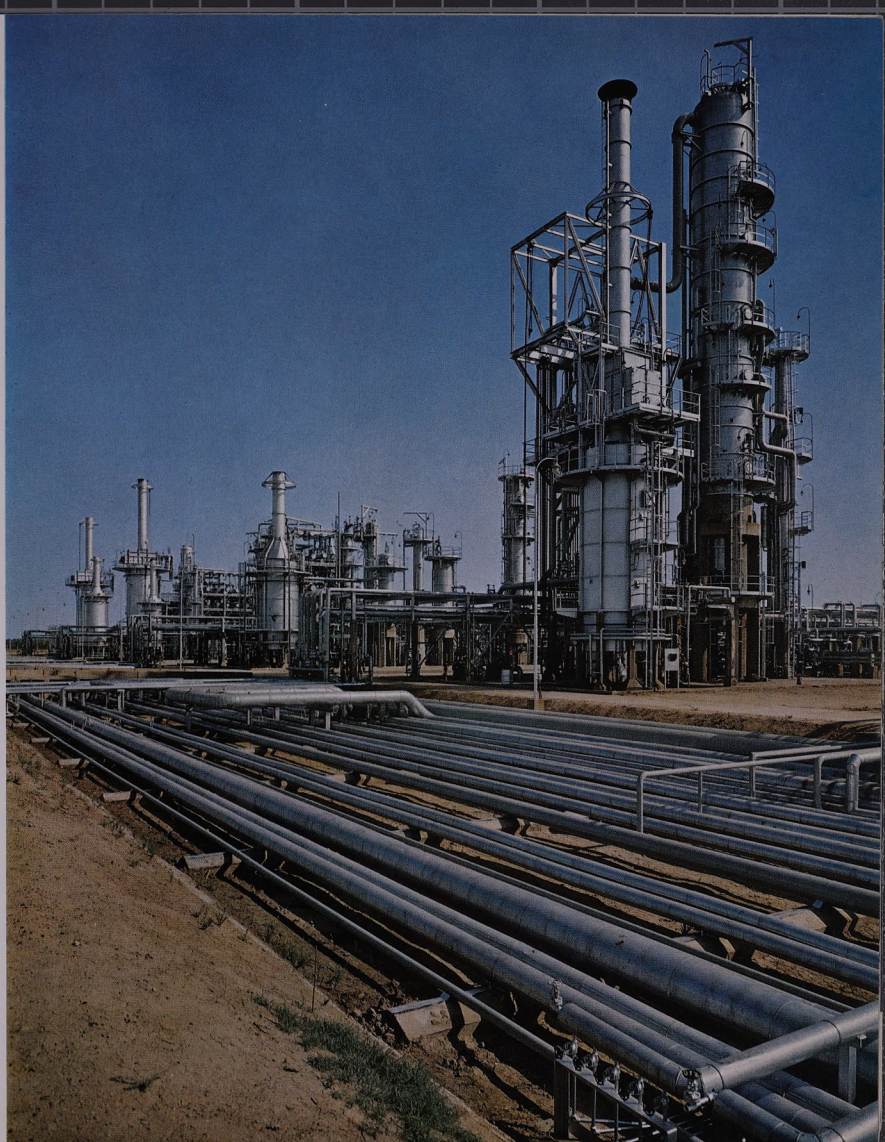
Pipe-way and process units
