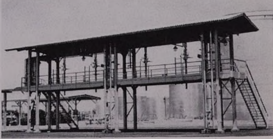
ASPHALT BLENDING AND FILLING UNIT
