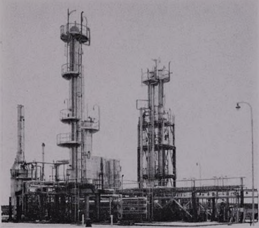
LUBE OIL HYDROFINISHING UNIT (745 BPCD)
