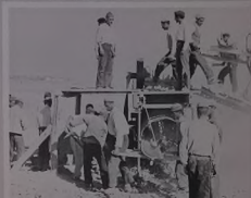
Rock crusher prepares ballast for the railway. Ballast will be stored nearby until embankments have settled sufficiently for its application. Although not seen, an adequate quantity of rails to extend the Iranian portion of the link from Sharafkhaneh to Kara Tepe Mountain, halfway to the Turkish border, is now in storage.
