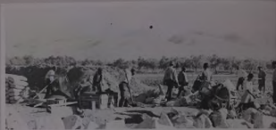
Laborers engaged in the construction of one of 219 culverts being built along the 40 kilometre section. Stone comes from a quarry nearby. The donkey carries fresh drinking water to workers.
