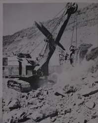
A giant excavator (above right) bites into a mass of rock and dirt at the side of one of twenty stations between Muş and Tatvan. It and the large dumper (left) building up an embankment are among 317 separate pieces of mechanical equipment kept in operation day and night throughout the construction season lasting from March until November.
