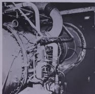
Rolls Royce Avon jet engine at the crude oil pumphouse.
