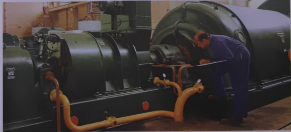
A gas turbo-alternator at Burgan Power Station.
