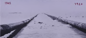
1945 Construction of a 12-inch crude oil pipeline from the Dammam field in Arabia to Bahrain was completed during the year, with 17 of its 94 miles running beneath the waters of the Persian Gulf. The pipeline was subsequently doubled.
